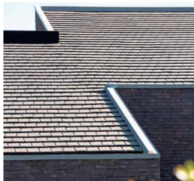
Dak met Koramic Migeon Vauban antraciet mat. Architect: Buedts & De Pape, Ertvelde
